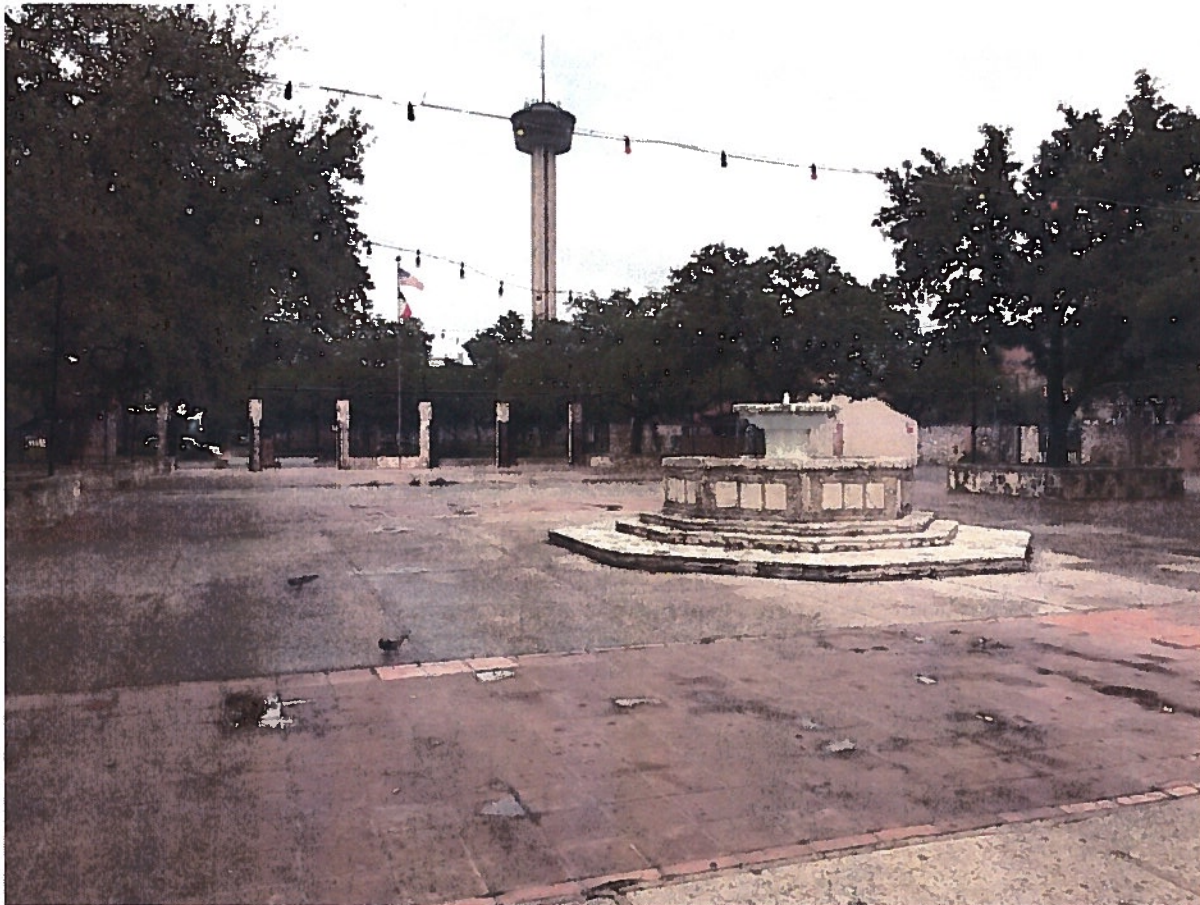
Figure 22. Poor paving and drainage conditions.
